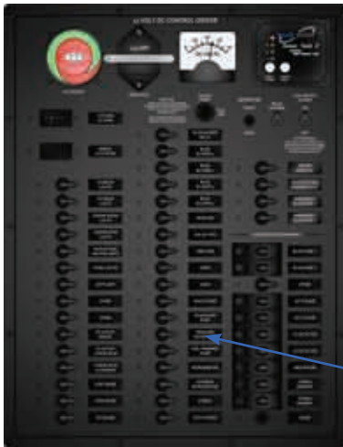
DC CONTROL PANEL
