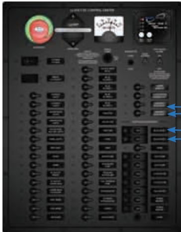
ITEM 2: AC CONTROL PANEL
