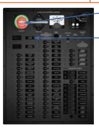
DC CONTROL PANEL
